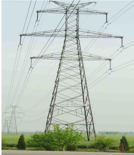
Figure 1.1 Transmission line tower
