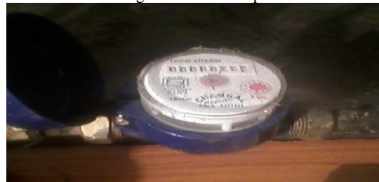
Figure 3.4: Flow Meter Arrangement
