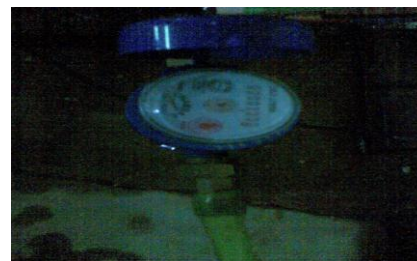
Figure 2.2: Water flow meter
