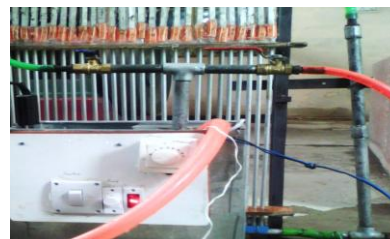
Figure 2.4: Electrical control panel
