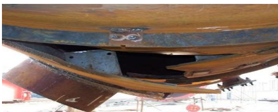
Figure: 1) Failure due to internal pressure
