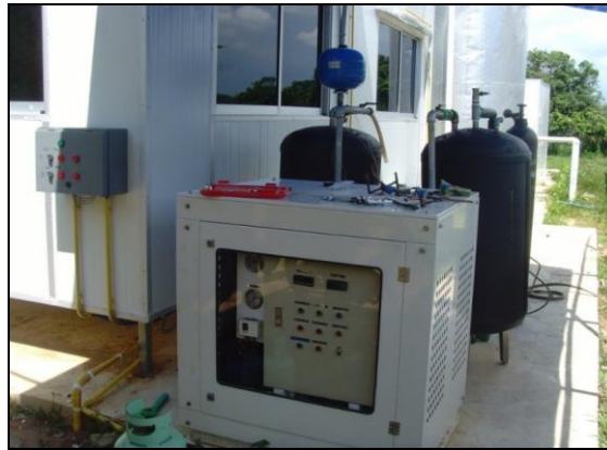
Figure 4. 10 kW of R-123 vapor compression heat pump.
