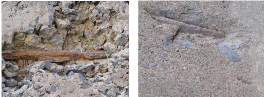
Fig. 1.1 Exposed reinforcement in piers due to spalling of cover
