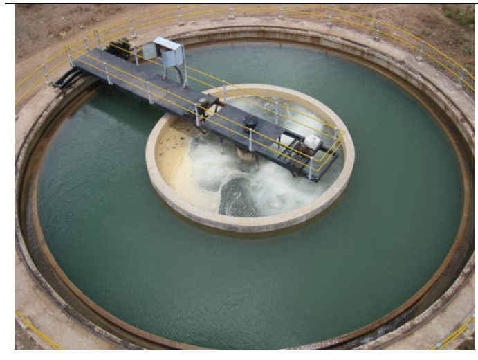
Fig: No.1 Sedimentation Tank
