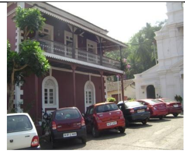
Fig. 8. Heritage Houses in dilapidated condition due to non maintenance.
