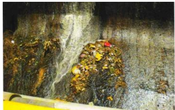
FIGURE.2 GARBAGE DEPOSITED BENEATH THE SPILLWAY
